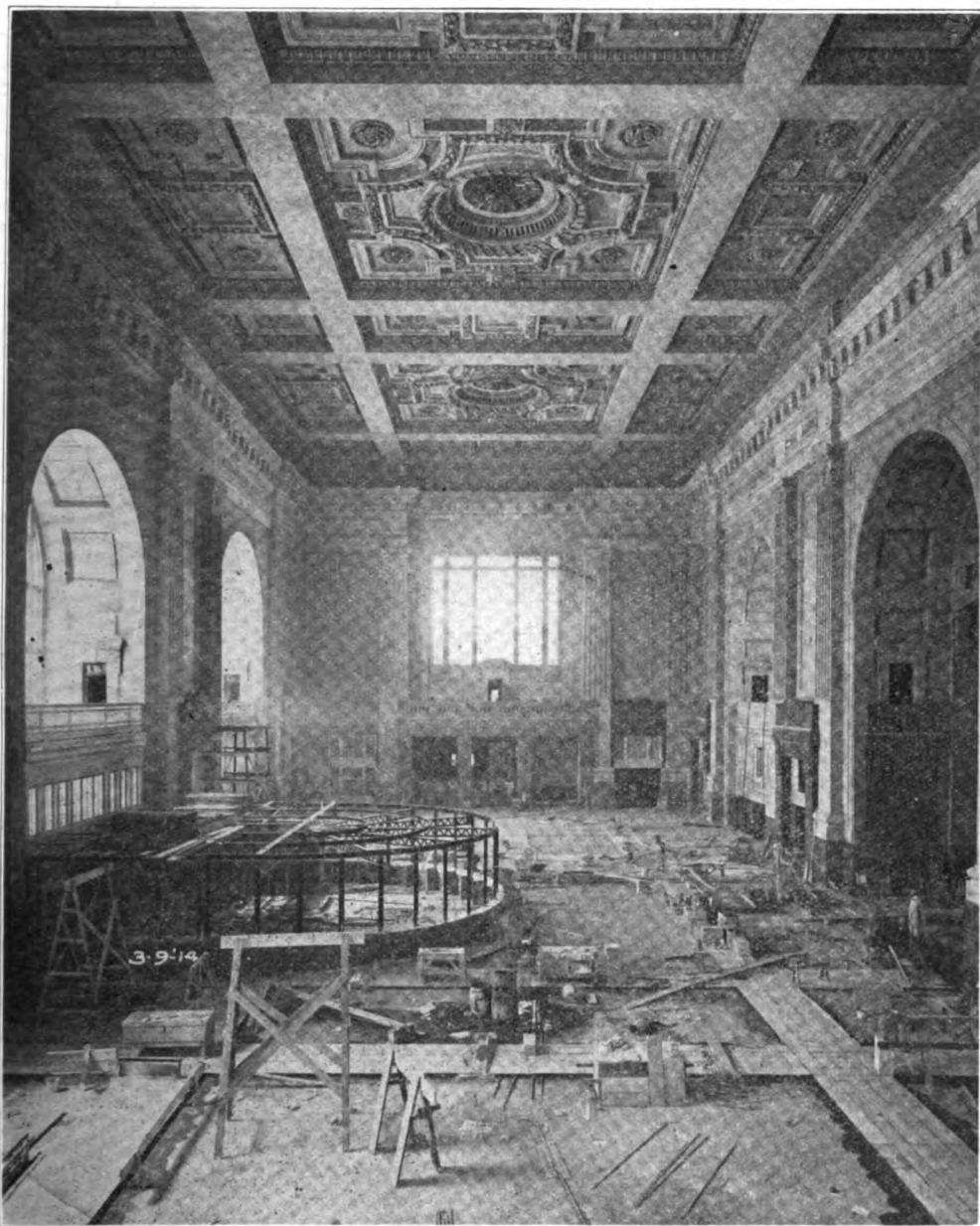
FIG. 5—WEST END OF GRAND LOBBY. ENTRANCE TO WAITING ROOM ON EXTREME RIGHT.
